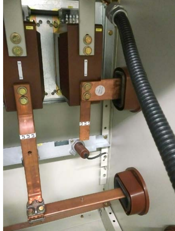
Defective capacitive insulator in 12 kV switchgear (see error pattern on the previous page)
