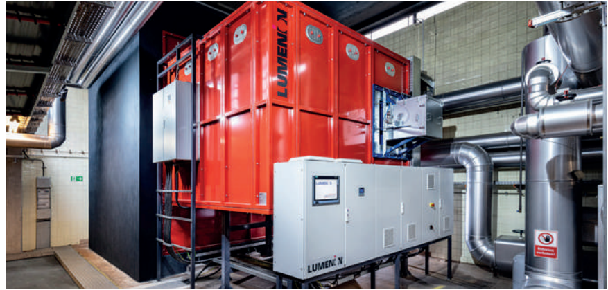
Storage unit integrated into a heating system of a residential complex in Berlin
