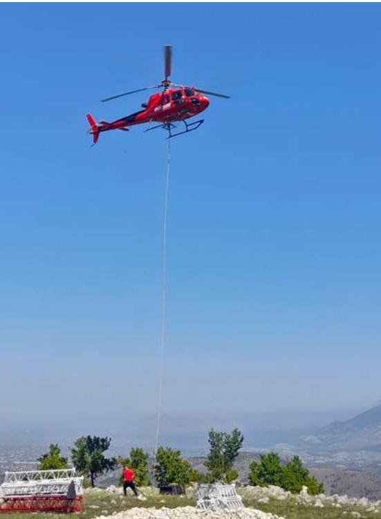
Installation of a wind met mast in difficult terrain with helicopter support
