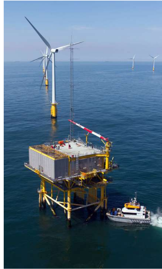
Offshore Substation Photo: halberg, stock.adobe.com
