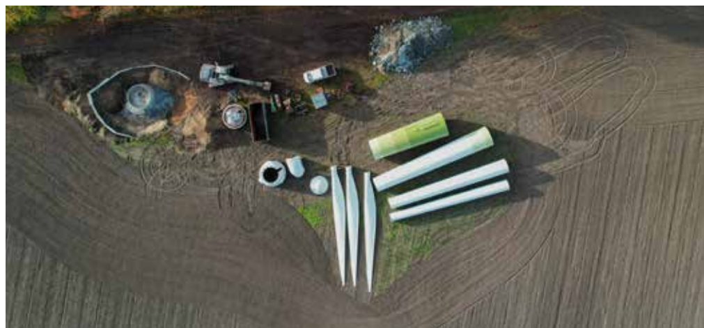
Elster wind farm: Dismantling of the 50 older Enercon E-40 units; temporary storage of the old systems. Photo by VSB Group.
