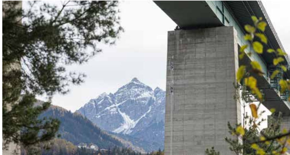
View of the Europa bridge with installed MOWEA turbines
