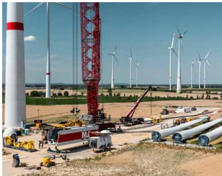
The aim of REZ' innovative concept is to minimise red tape and costs even for major projects.
