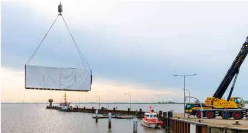
Moving the corrosion protection metrology container from BAM TTS to the Eider barrage location Source: BAM
