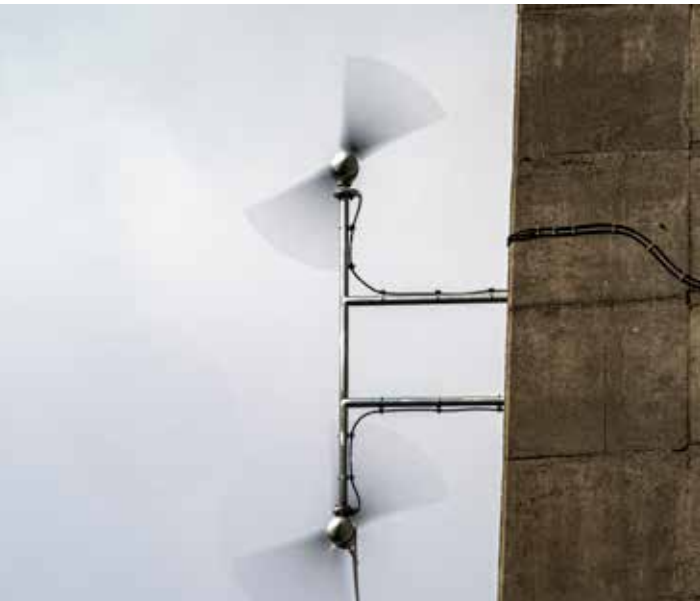
MOWEA wind turbines on the Europa bridge
