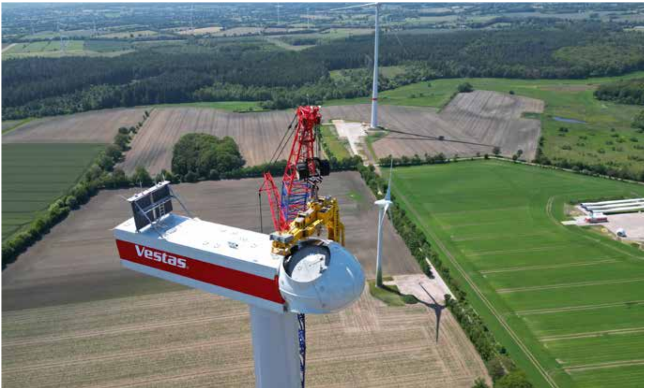
Installation of the nacelle at the wind farm Reher in June 2023 (Photo J.Weidkamp)
