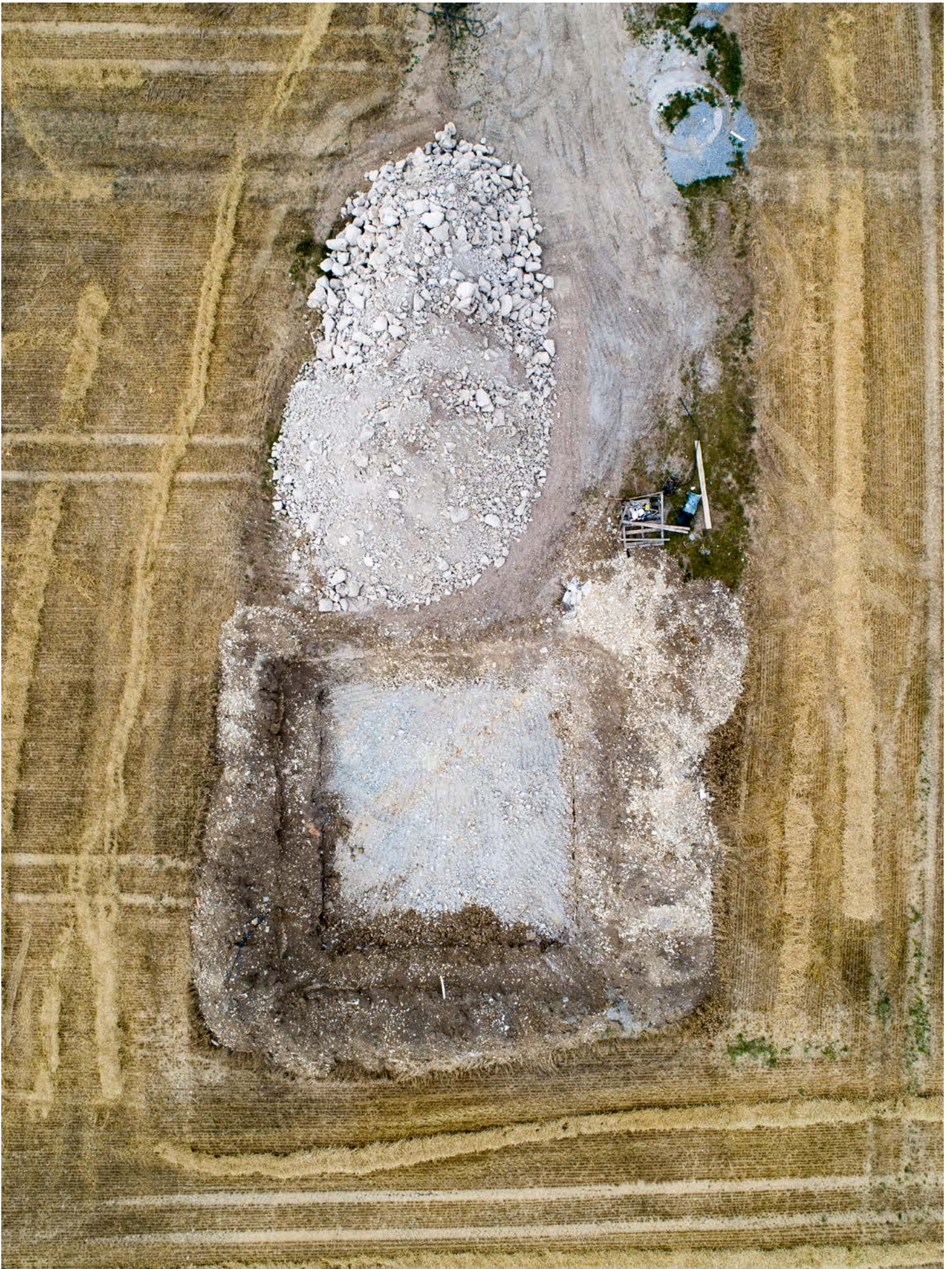
The broken up foundations of a wind turbine at Elisenhof/Meerhof wind farm. Photo: Ulrich Mertens
