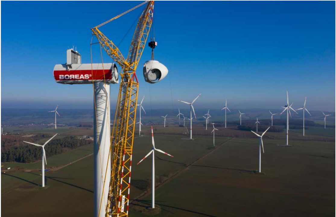
Erecting a V150-4.2 MW Vestas turbine at Neukirchen wind field in Thuringia. Photo: Jan Oelker
