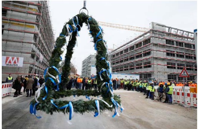
The topping-out crown for the first module of the Siemens Campus Erlangen has been set. Photo: Siemens AG
