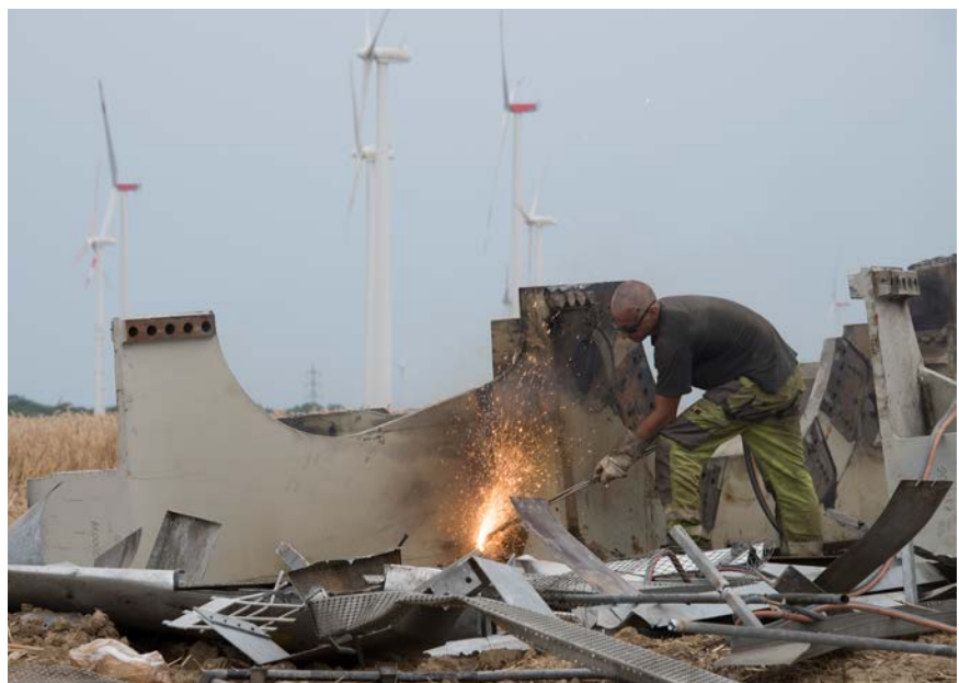
The dismantling of a wind turbine at Eisenhof/Meerhof wind farm. . Photo: Ulrich Mertens
