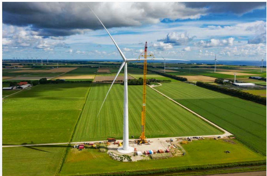
Prototype of the E-160 EP5 in the Wieringermeer wind energy test field in the Netherlands Photo: Klaas Eissens
