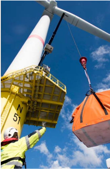
Service work at Nordsee One wind farm. Material is hoisted from the WINDEA Four to the work platform. Photo: Ulrich Mertens
