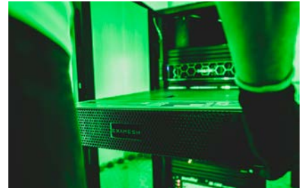
Right: The installation, operation and maintenance of the EDC is carried out by ExaMesh.
