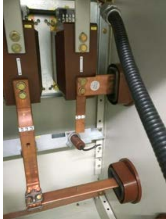
Defective capacitive insulator in 12 kV switchgear (see error pattern on the previous page)
